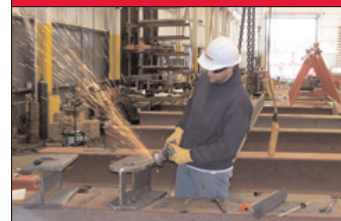
John Declute, our certified welder, prepping an end connection for a tie in strut.
